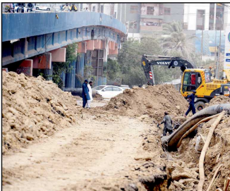
Karachi: Local Government Department Supervises New Drinking Water Lines Construction at Rashid Minhas Road Near NIPA Chowrangi, Karachi.
