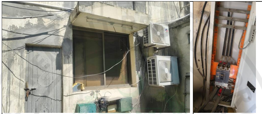
Control Room for Main Building
