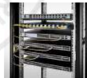
Figure 5. Switches mounted in a Rack
